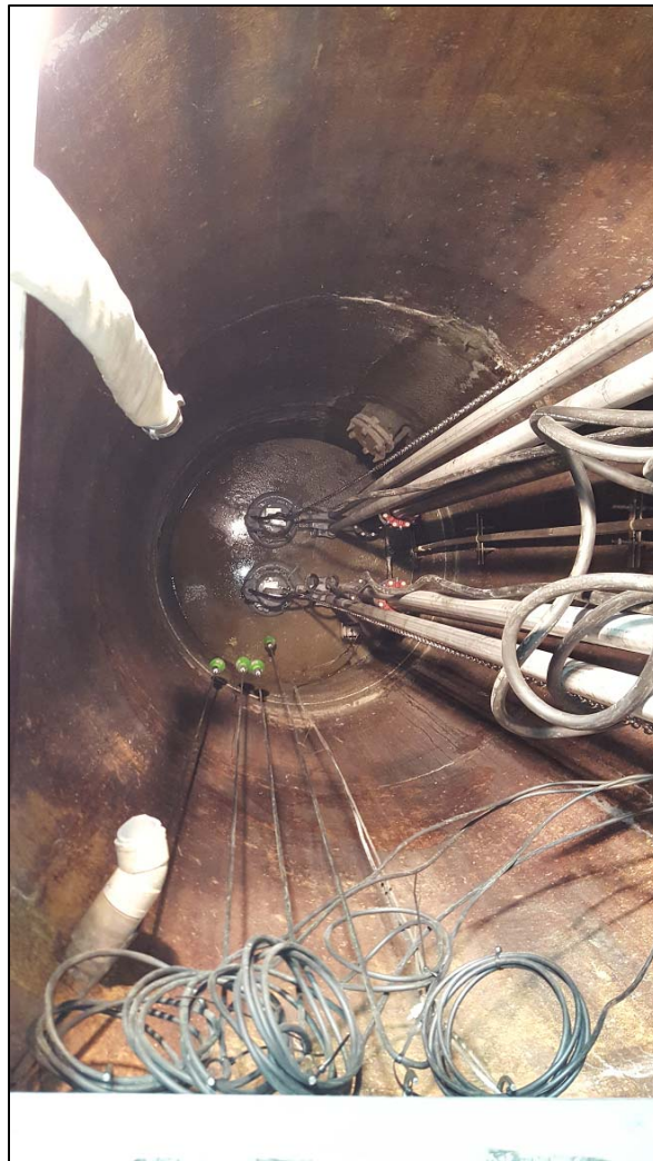
New pumps, pump rails, discharge piping, and control floats at the Cantova sewer pump station.
