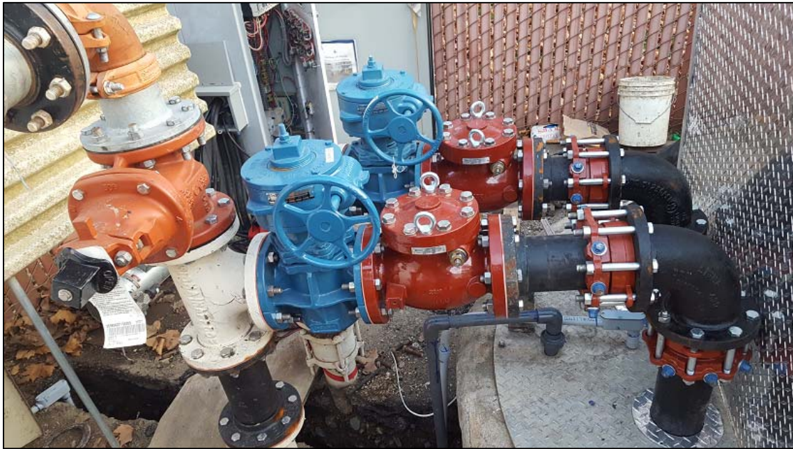
New valves and check valves on discharge of new pumps
