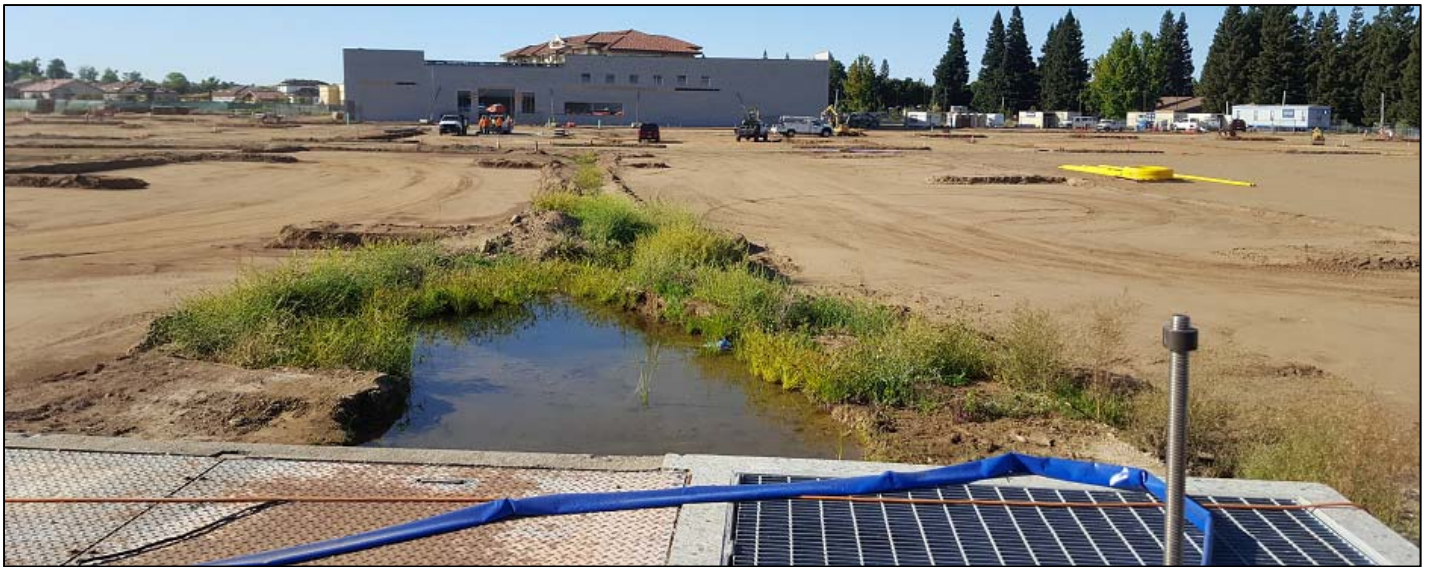
Photo from Cosumnes Irrigation Association diversion box looking towards Bel Air store being constructed
