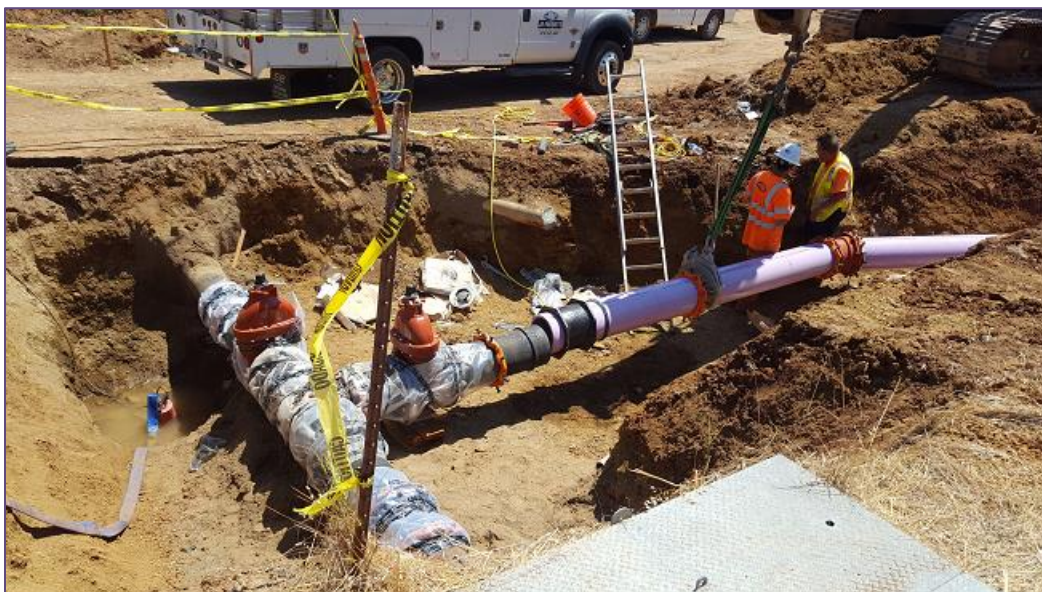
Photo of point of connection from recycled water line going to Bass lake to Murieta Gardens/Commercial areas.
