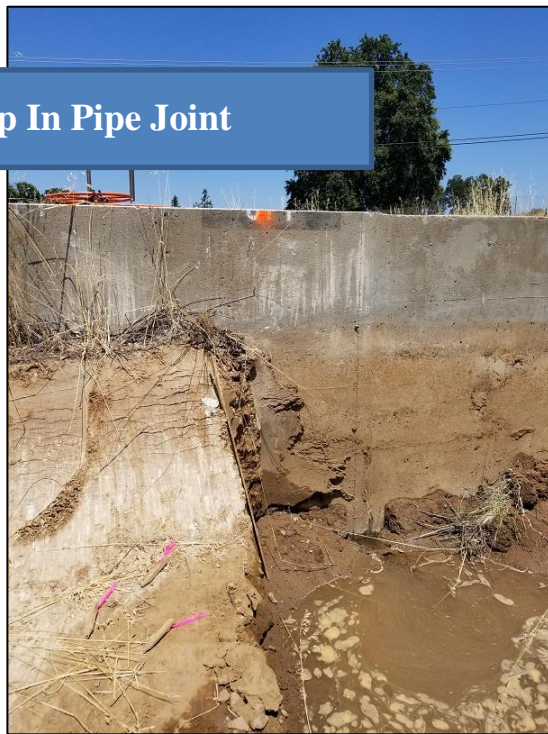
July 7, 2019 photo showing leaking
