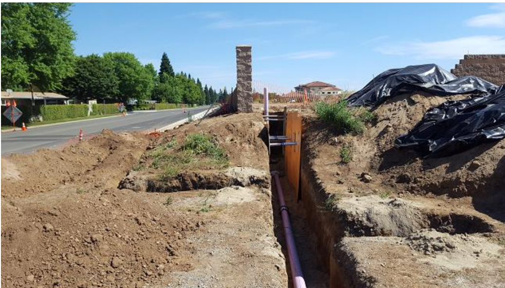
Photo of 6 inch recycled water line running towards Cantova Drive from Murieta Gardens Lot 66
