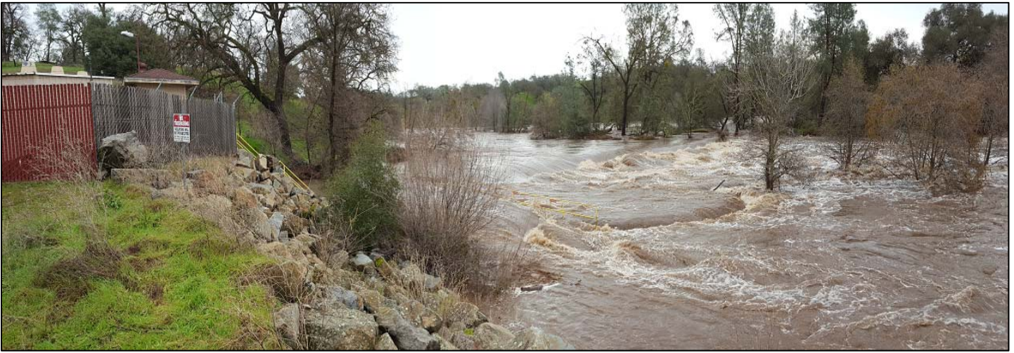
Granlees Diversion Structure & Cosumnes Irrigation Association (CIA) Ditch underwater from high river flows, upstream view.
