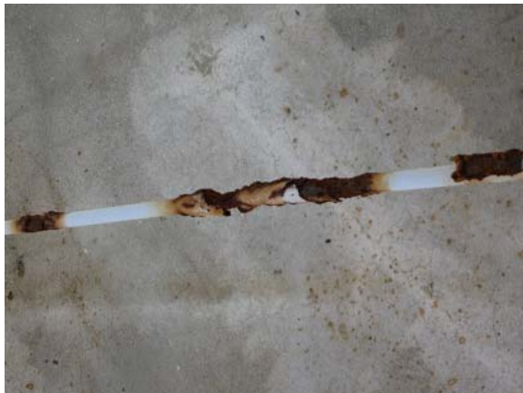
Typical tie-rod support inside DAF unit
