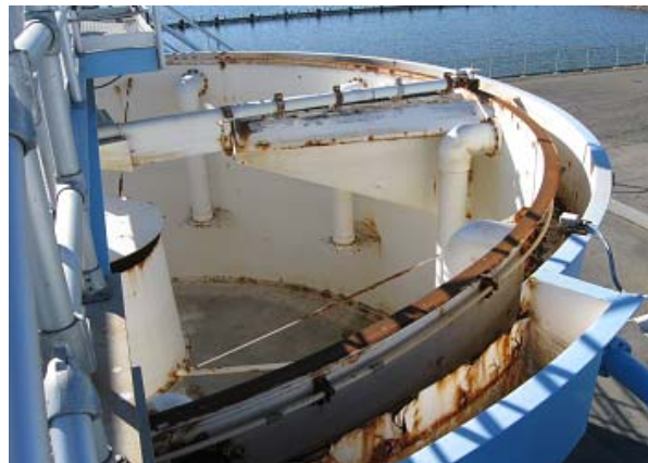
Deteriorated overflow weir, scum trough, & other areas of concern
