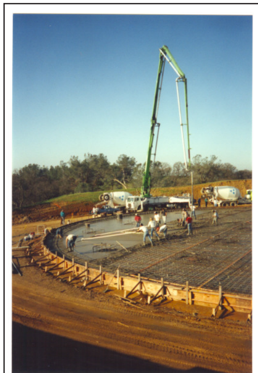
Construction for the 3 million gallon concrete water storage tank east of Rancho Murieta in 1989.
