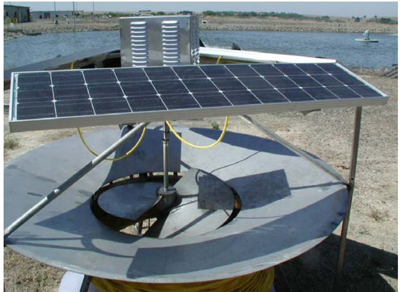
This solar bee increases efficiency and lowers the cost of running the aerators at the wastewater plant.
