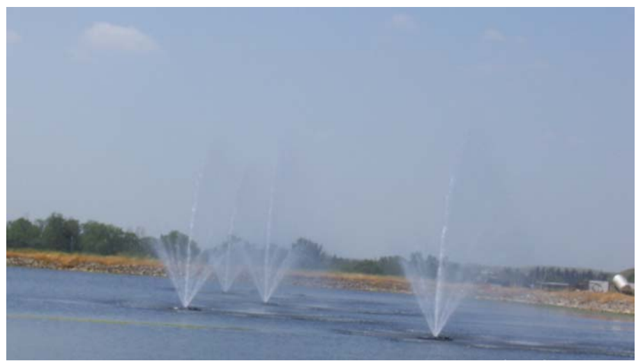
Aeration fountains at the wastewater treatment plant.
