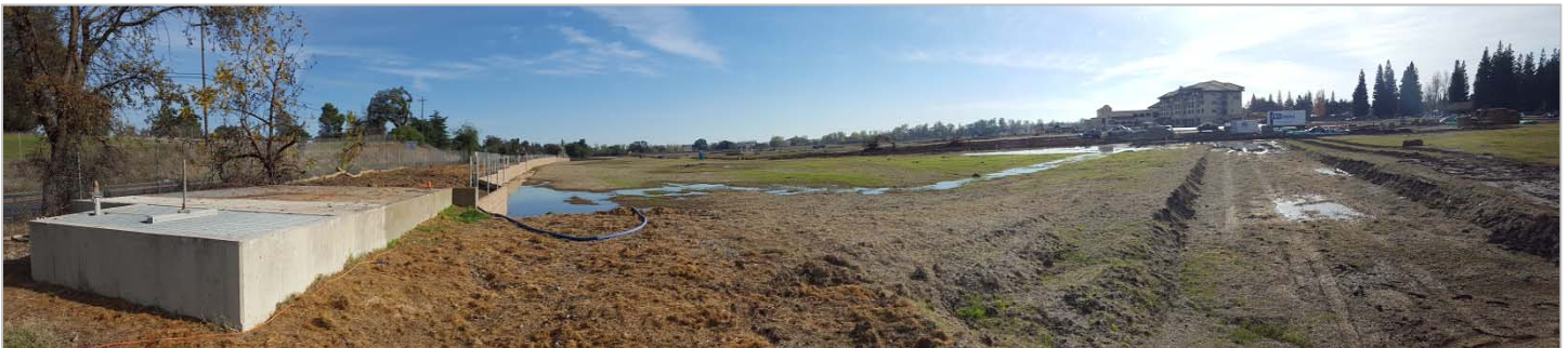
Photo of the lowered diversion structure and site area for the Murieta Marketplace with Murieta Inn in the background.
