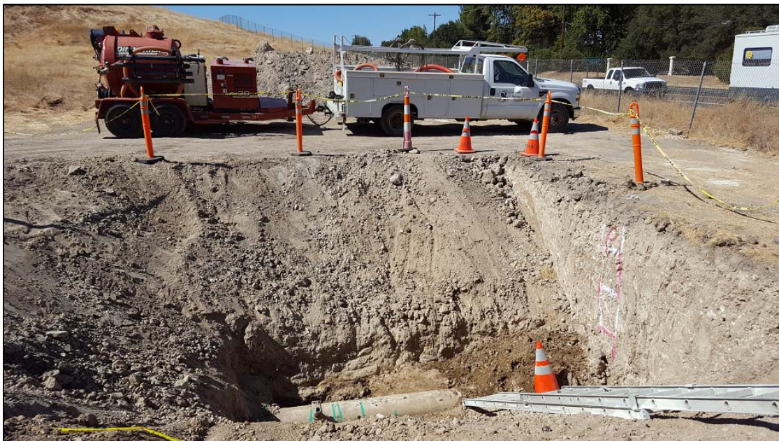
Photo of 12 inch force main pipeline to possibly be used for future conveyance of recycled water.
