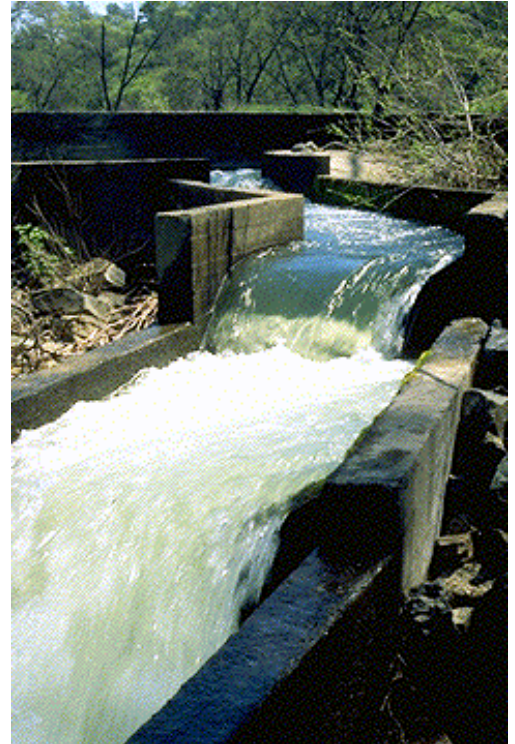
Fish ladders at Granlee Dam
