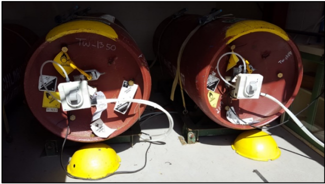
Ton cylinders of chlorine gas
